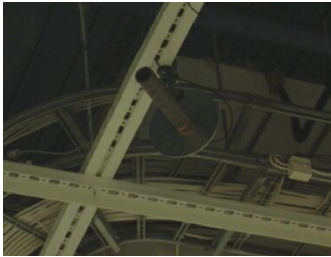
Fig. 2. The pseudolite antenna attached to the ceiling of the Exhibition Hall 2
